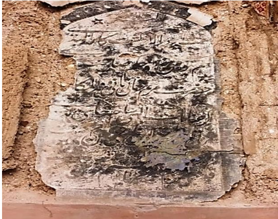
Fig. 4 Deteriorating calligraphy and corroded bricks of the Maryam Zamani Mosque.
