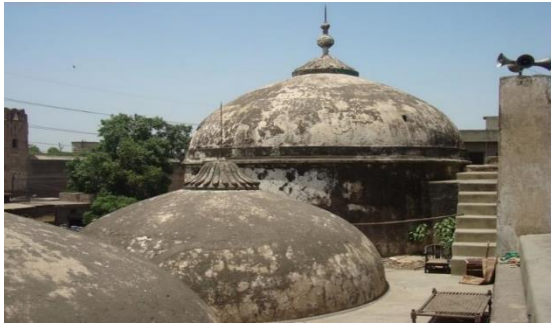
Fig. 1 Modern addition and use of Portland cement instead of lime mortar
