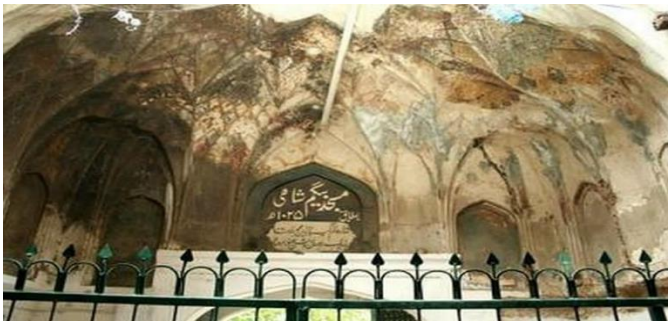
Fig. 5 Repairing of original lime plaster with modern cement, fixation of iron pipe in original structure for electrification and provision of ugly iron grill.
